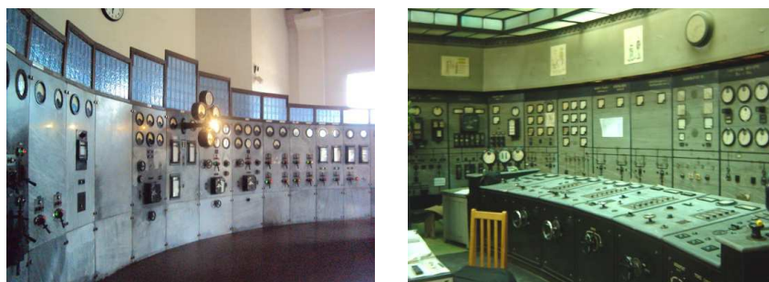
Figures 16,17. A comparison between the control board of Fábrica de la Luz (Ponferrada, Spain), former plant and control board of the electric plant of the Anina mines ensemble (Source: photos by the author, 2013/2007)
