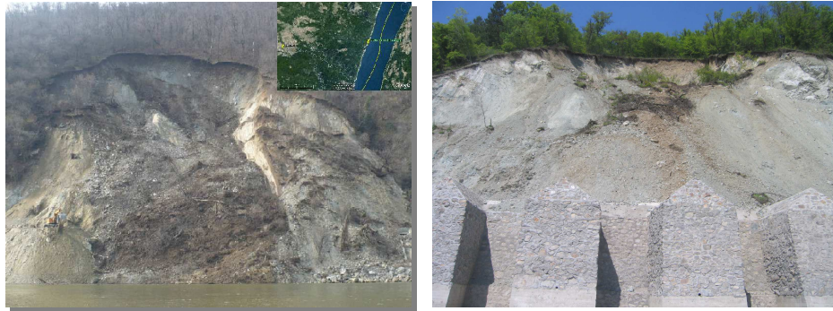
Fig. 8. Landslides which affected the national road (left) and the slope protection works (right) in Liubotina – Danube Gorge
