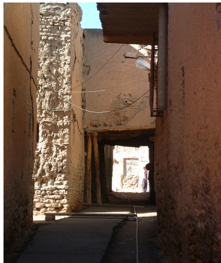
Fig. 6. Destruction of the traditional houses destroyed (Source: The author in 2007)
